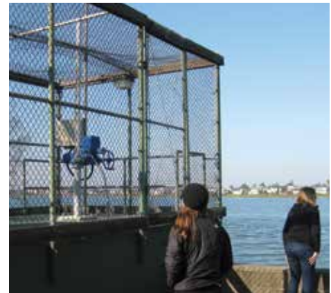
Bay Farm Isle pump station, one of hundreds of aging facilities around the region used to keep our communities and shorelines dry. Many are under-sized, at capacity, and at the end of their service lives. To cope with SLR and storms, they need upgrades, maintenance, and back up power. Photo from archives.
