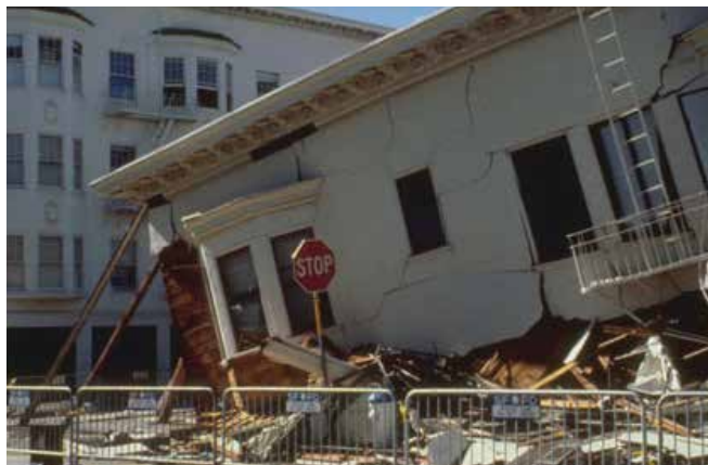
Liquefaction impacts in the Marina District from the 1986 Loma Prieta quake. Photo USGS
